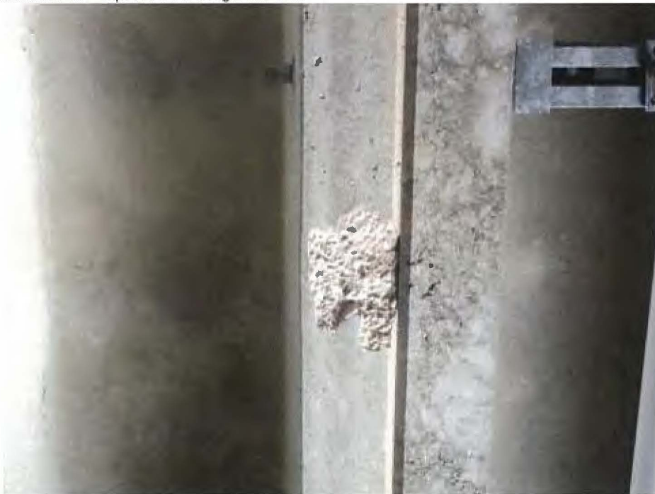
Photo 25: Typical spall/delamination with exposed steel along Beam 5-12
